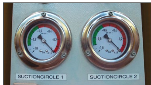
Dual circuit vacuum system
